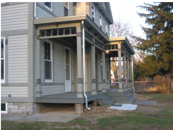
[AFTER - Vanguard worked with new owners to restore the roof and porch back to original. The tin roof is made of 14" x 20" sheets of terne, interlocked and soldered.]
