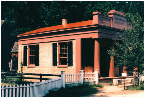
[New Terne Roof, Locked And Soldered 14 X 20" Sheets, (1840) Thompson Bank. Old Sturbridge Village, MA]
