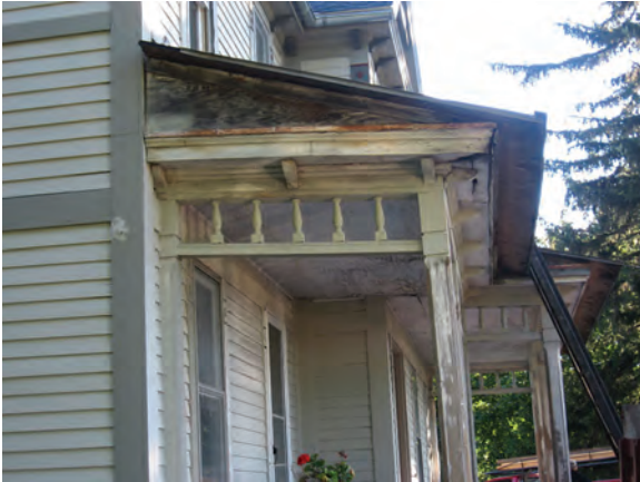
[BEFORE - Years of neglect led to spanning the tin roof and built-in gutter on this 1880 Folk Victorian.]
